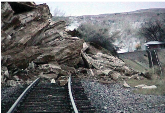
FIGURE 3 Rockfall, Thermopolis, Wyoming, 2002. (Photo credit: D. McCulloch.)
