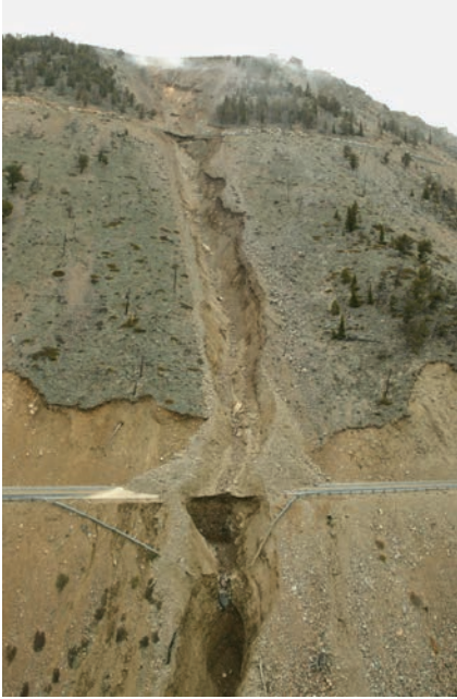
FIGURE 5 Debris flow, May 2005, Beartooth Highway, Montana. (Photo credit: Montana Department of Transportation.)
