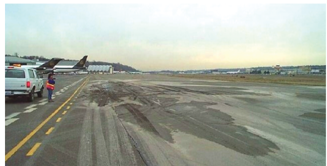
FIGURE 4 Nisqually Earthquake, February 2001, sand boils, Boeing Field Taxiway, Seattle, Washington. (Photo credit: M. Anderson.)
